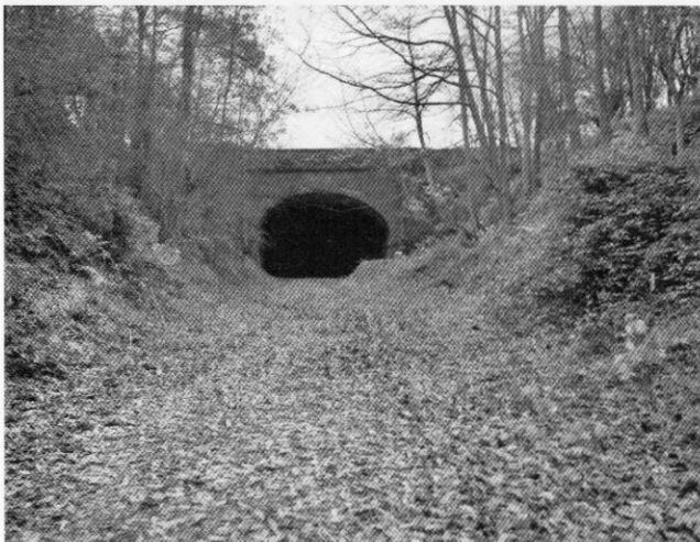
The south portal of Bourne Park tunnel in 1982. Taken from the same view point as above. Photo by Nick Catford
